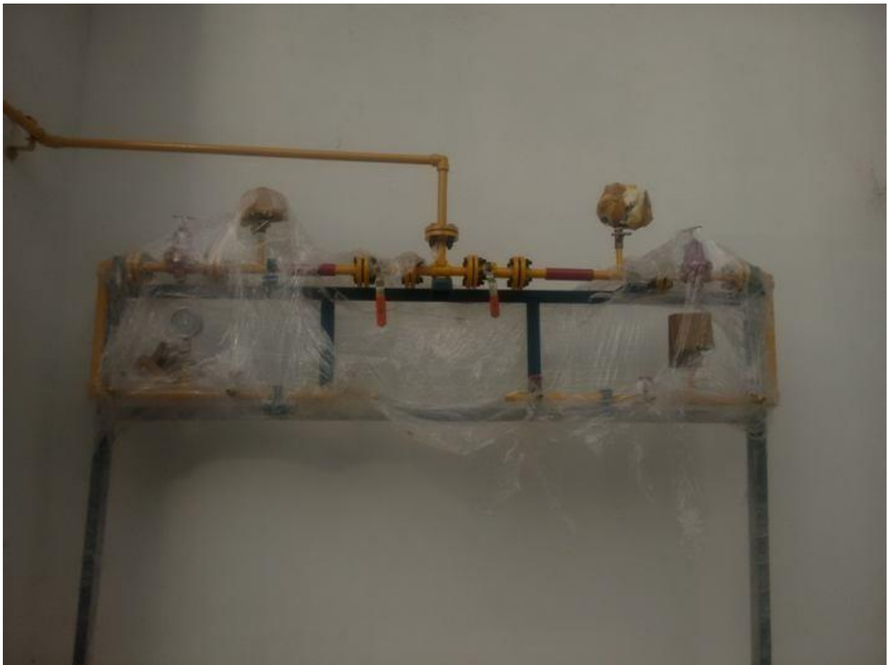
2 x 3 cylinders LPG Manifold. Griffith Foods Pvt. Ltd., Doddaballapur.
