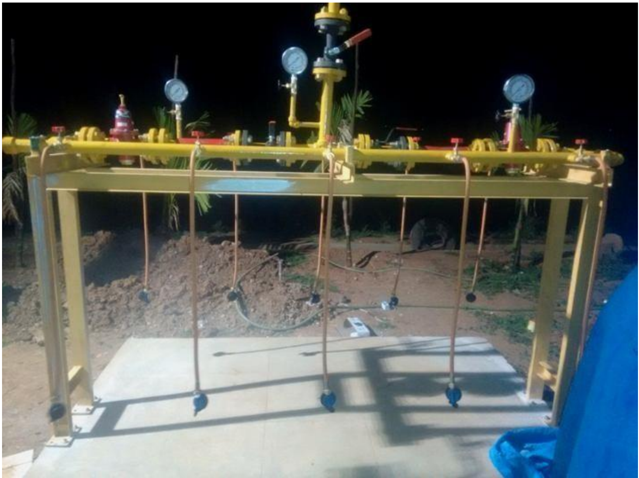
2 x 5 cylinders LPG Manifold. Griffith Foods Pvt. Ltd., Doddaballapur.
